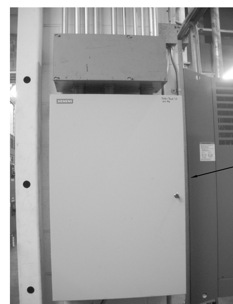
6 PHOTO RECORD - EXISTING EMS CONTROL PANEL E2.14 SCALE: NONE
