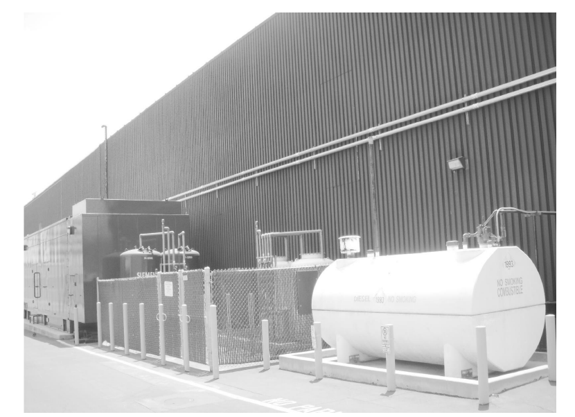
9 PHOTO RECORD - EXISTING "THE BIG RED" STANDBY GENSET E2.14 SCALE: NONE
